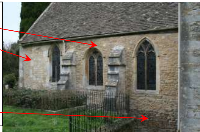
Fig 301 – south wall of the nave. Buttresses to support south wall. 3 Decorated Gothic windows (early C14 th ). Note blocked window at west end (see internal photo) (possible external entrance to 19 th C gallery). Note stonework – freestone coursing especially below eastern most window. Darker stone suggests it was level below ground until C20 th .
