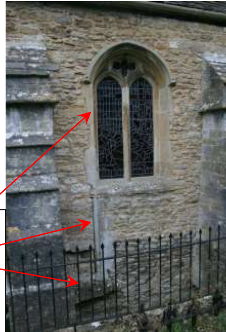
Fig 303 – Decorated Gothic window restored in 19 th C. Note door post column below window (no other evidence of door). Bedded on a large protruding stone block (doorstep?).
