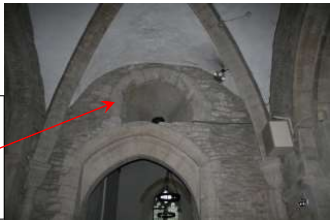
Fig 327 – South wall of tower crossing with upper Norman window and later arch into south transept. Late C12 th groined ceiling on Romanesque capitals.
