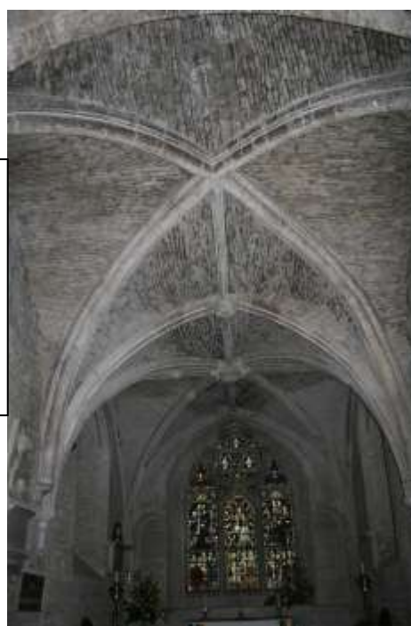
Fig 324 – Groined chancel roof with exposed rubble inbuilt (late 19 th early 20 th C ‘scraping’ ref SPAB [society for the protection of ancient buildings – scrape/anti scrape controversy]).
