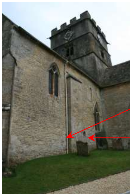
Fig 308 – North wall of chancel. Shows successive building lifts in the stonework with shallow buttress. Possible crypt below?
